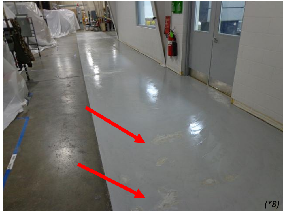
Concrete walking surface in a facility. Note the irregular areas where the potential for slips or trips are present.
