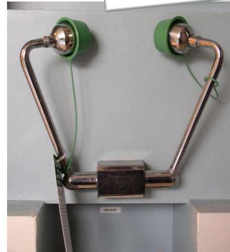
Eye wash station (*10)
